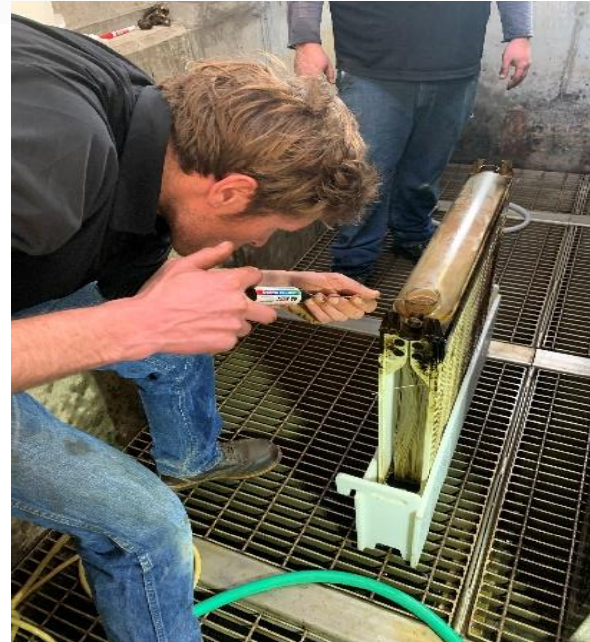
Logan makes membrane repairs right before the start of ECWC's busy season.
