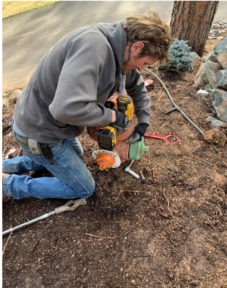
Logan removing a fire hydrant bonnet to access the internal stem, which was removed and replaced.
