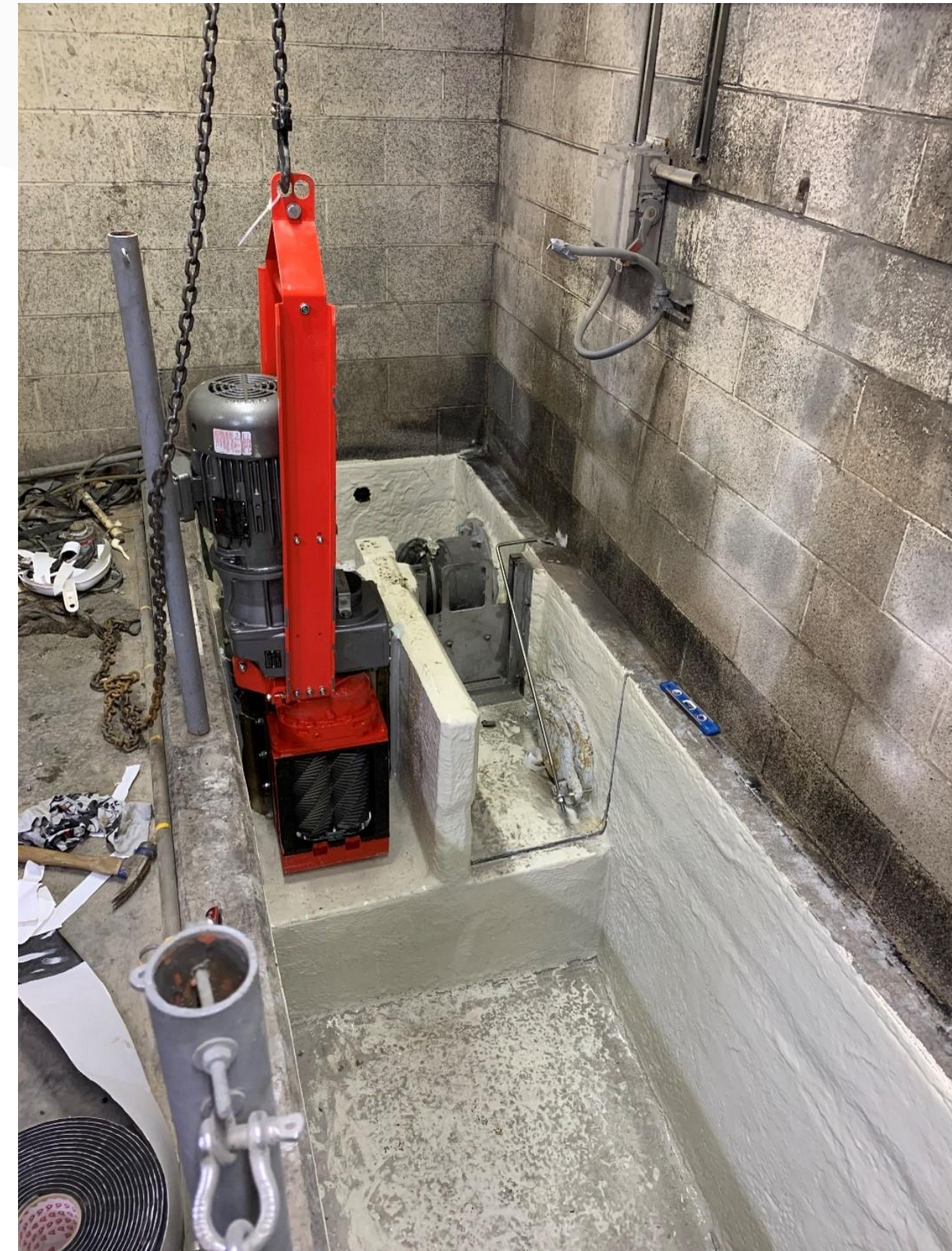
New grinder at the wastewater treatment plant headworks.
