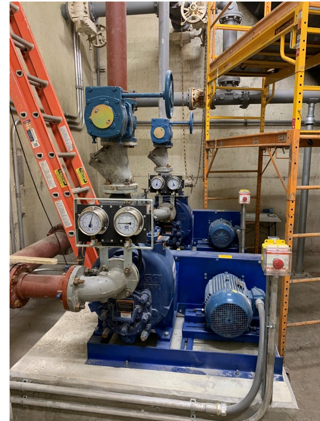
New sludge pumps in the wastewater treatment plant.
