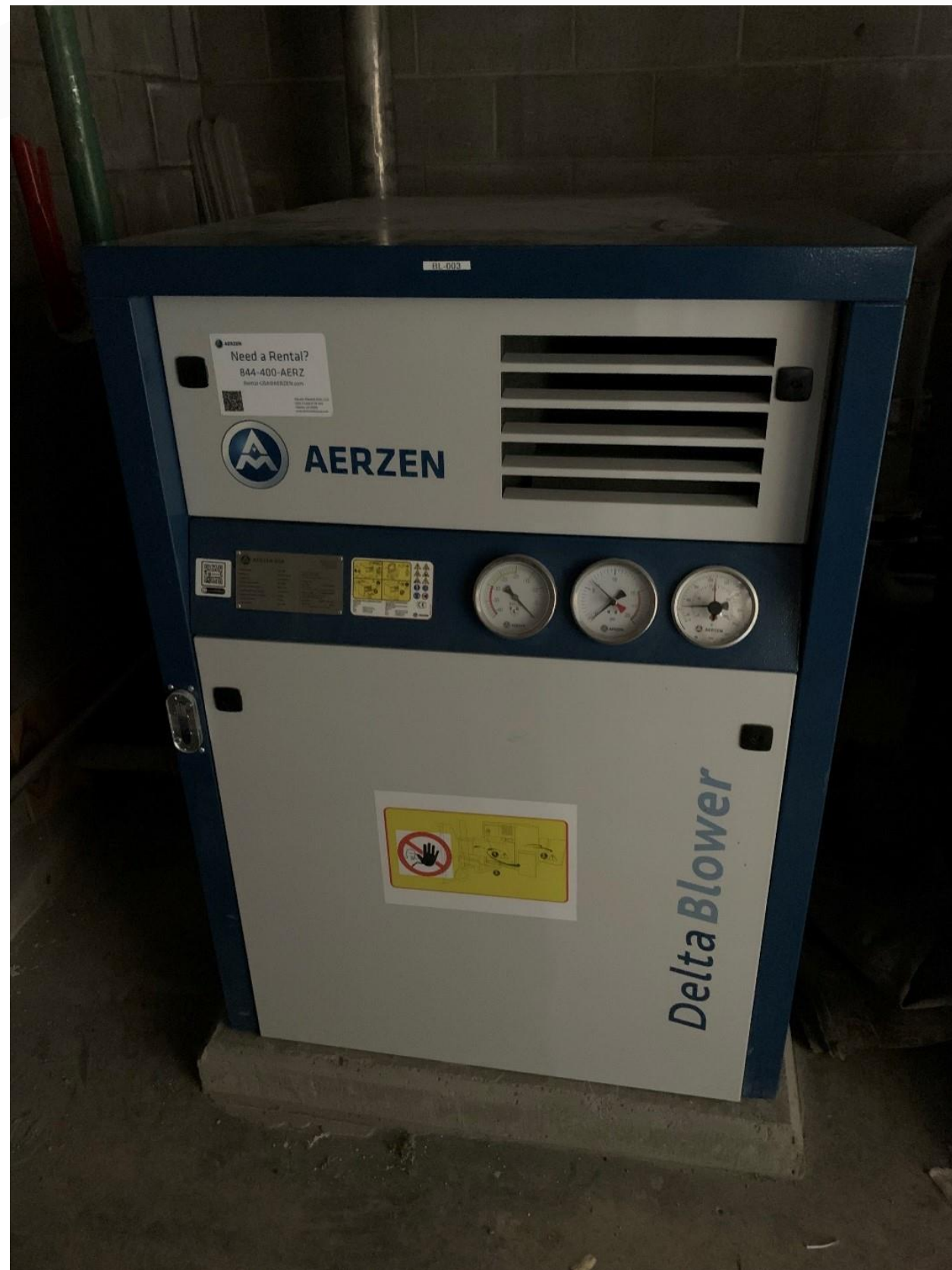
One of the new Aerzen blowers that provides air to the aeration basin diffusers. These new blowers are quieter and more energy efficient than the previous blower.
