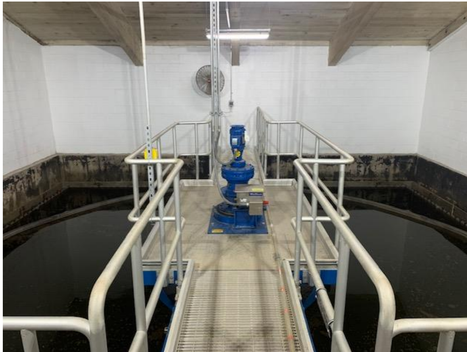
Figure 1: New Clarifier at Wastewater Treatment Plant
